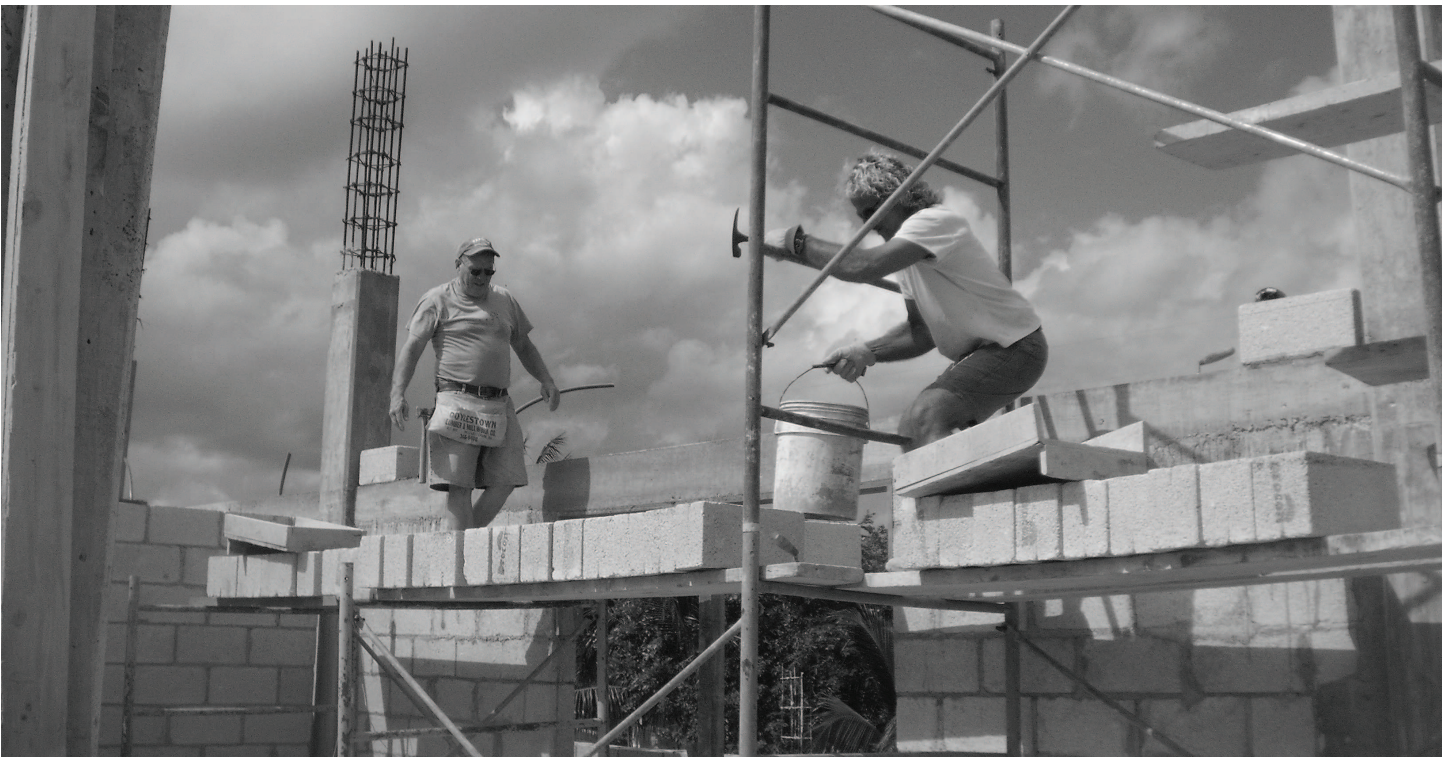
On the scaffolding, Rick Stoker (foreground) and another volunteer work with roof blocks
